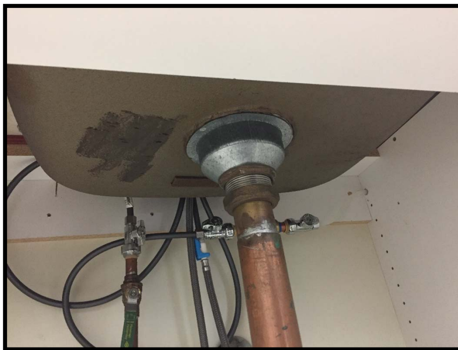
Photograph 1: Asbestos-Containing Gold Sink Undercoat.
