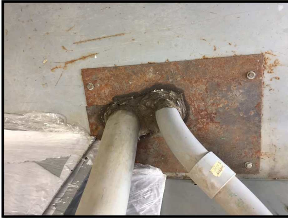
Photograph 1: Asbestos-Containing Grey Firestop.
