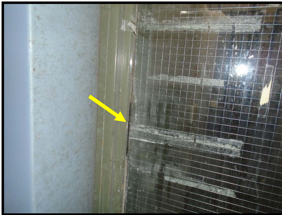
Photograph 1: Asbestos-Containing Black Window Glazing.
