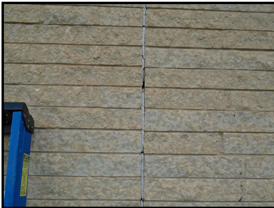
Photograph 2: Asbestos-Containing Grey Expansion Joint Caulking.
