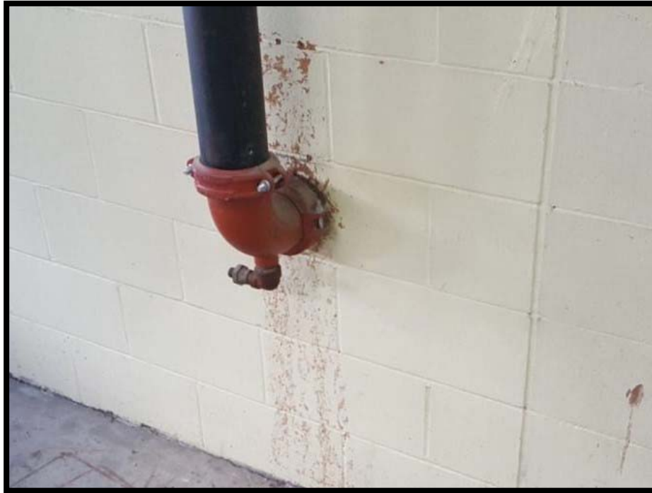
Photograph 1: Block Wall with Potential Asbestos-Containing Loose-Fill Vermiculite Insulation.
