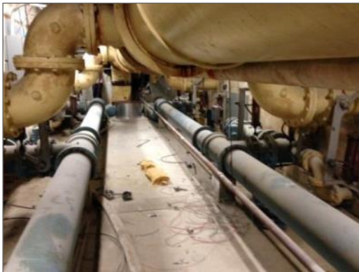
Photo 1 – View of lead based paints in the pipe gallery.
