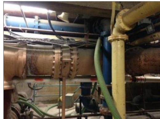
Photo 2 – view of various lead based paint in the pipe gallery
