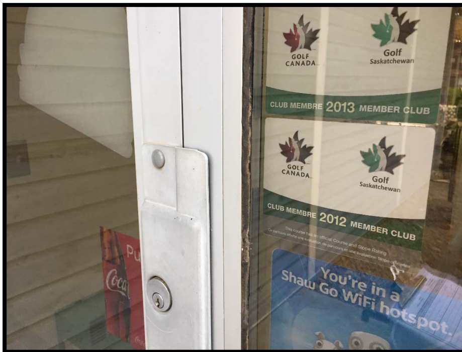
Photograph 4: Asbestos-Containing Black Exterior Window Caulking.
