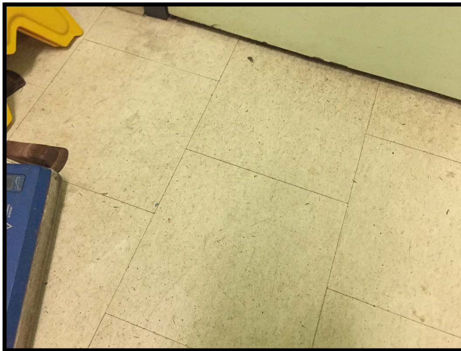
Photograph 1: Asbestos-Containing 12"x12" Off-White Floor Tile with Black Flecks.
