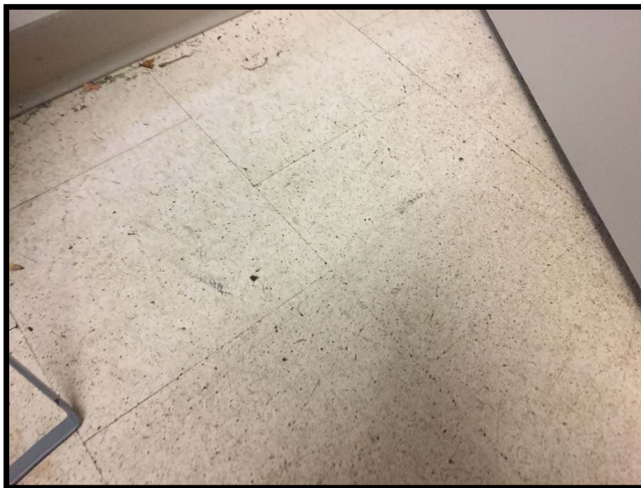
Photograph 2: Asbestos-Containing 12"x12" Off-White Floor Tile with Black Dots.
