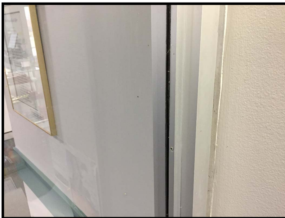
Photograph 3: Asbestos-Containing Black Interior Window Caulking.
