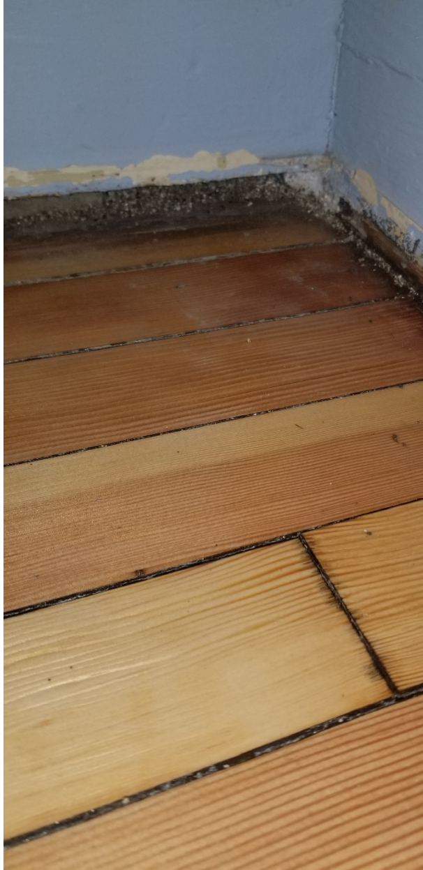
Photo 006- Vermiculite draining from wall in upstairs bedroom.
