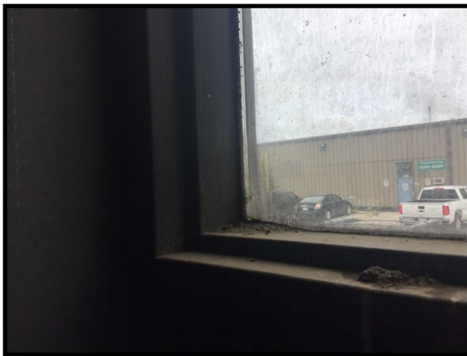
Photograph 1: Asbestos-Containing Black Window Caulking.
