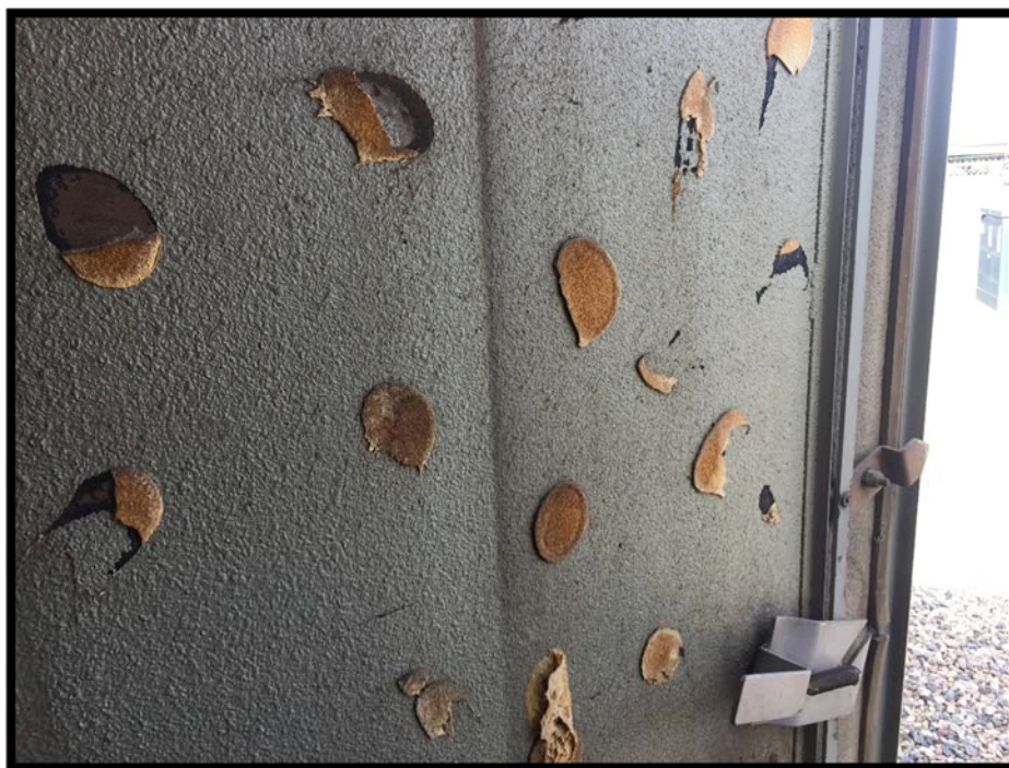
Photograph 1: Asbestos-Containing Wall and Ceiling Mastic.
