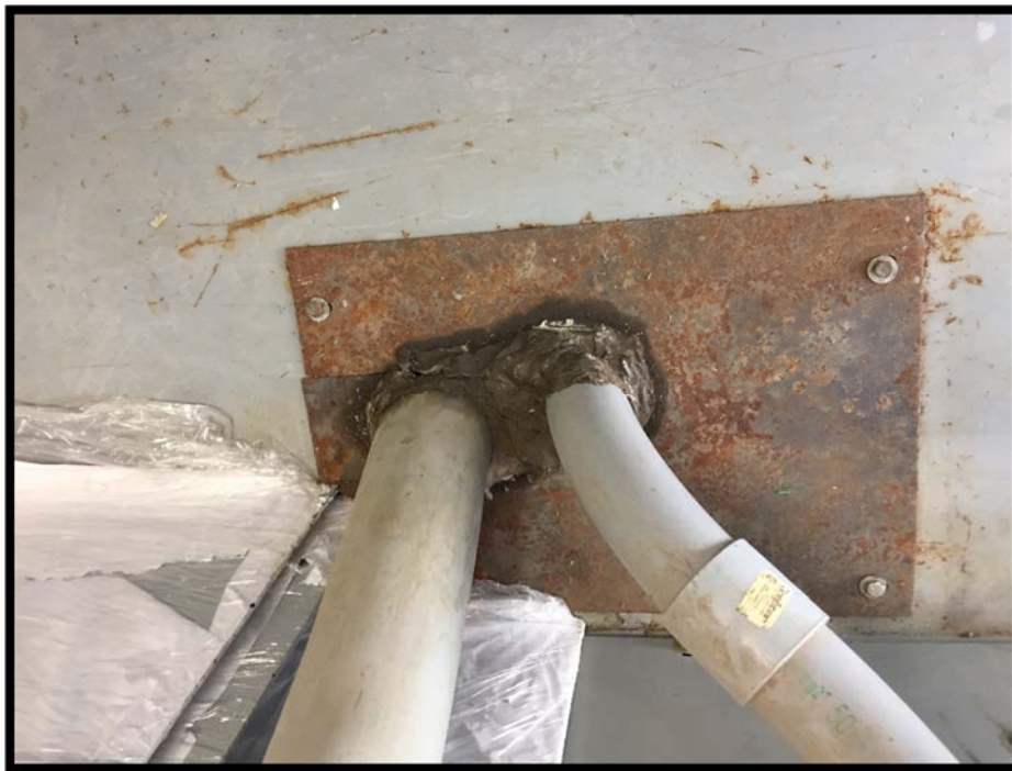
Photograph 1: Asbestos-Containing Grey Firestop.
