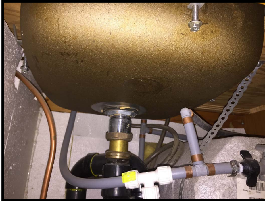
Photograph 1: Asbestos-Containing Gold Sink Undercoat.
