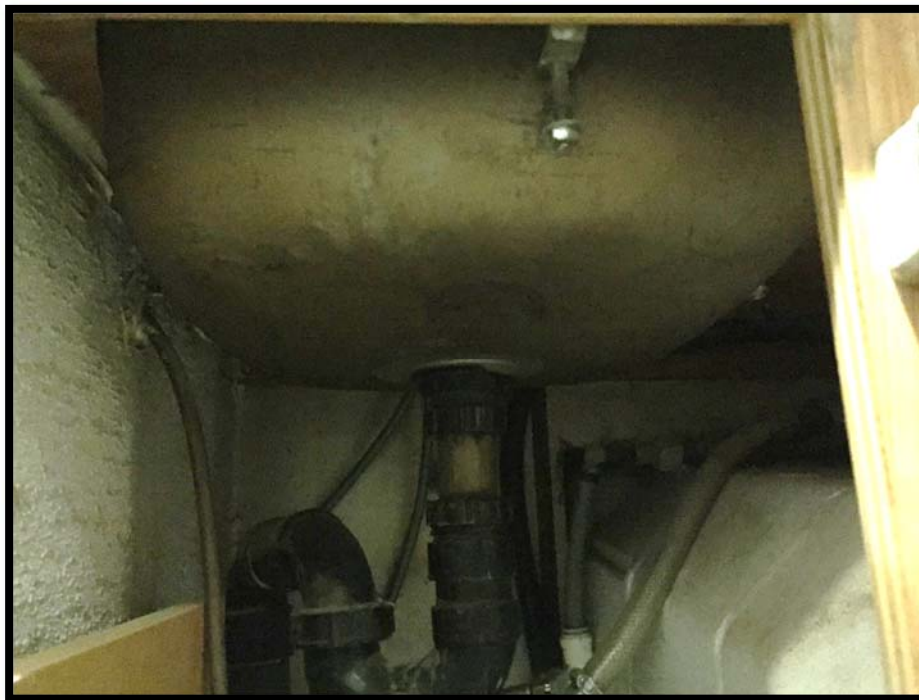
Photograph 1: Asbestos-Containing Gold Sink Undercoat.
