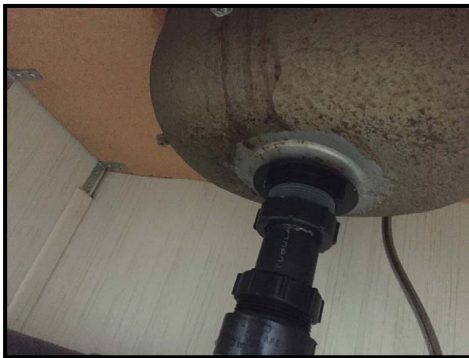
Photograph 1: Asbestos-Containing Silver Sink Undercoat.
