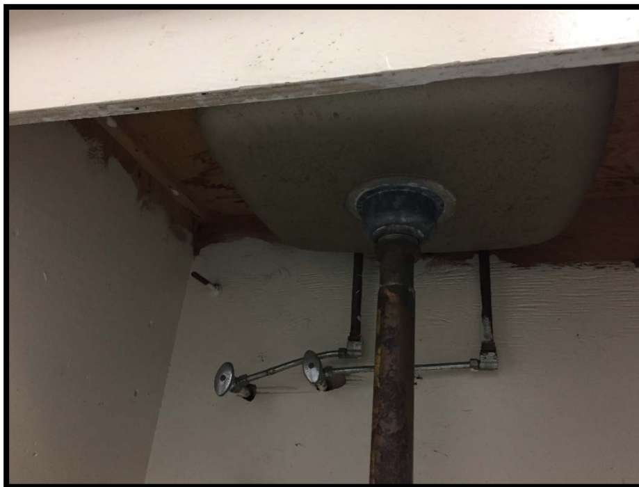
Photograph 2: Asbestos-Containing Silver Sink Undercoat.
