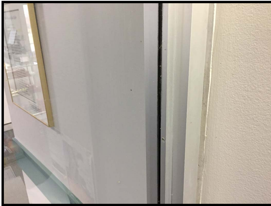
Photograph 3: Asbestos-Containing Black Interior Window Caulking.
