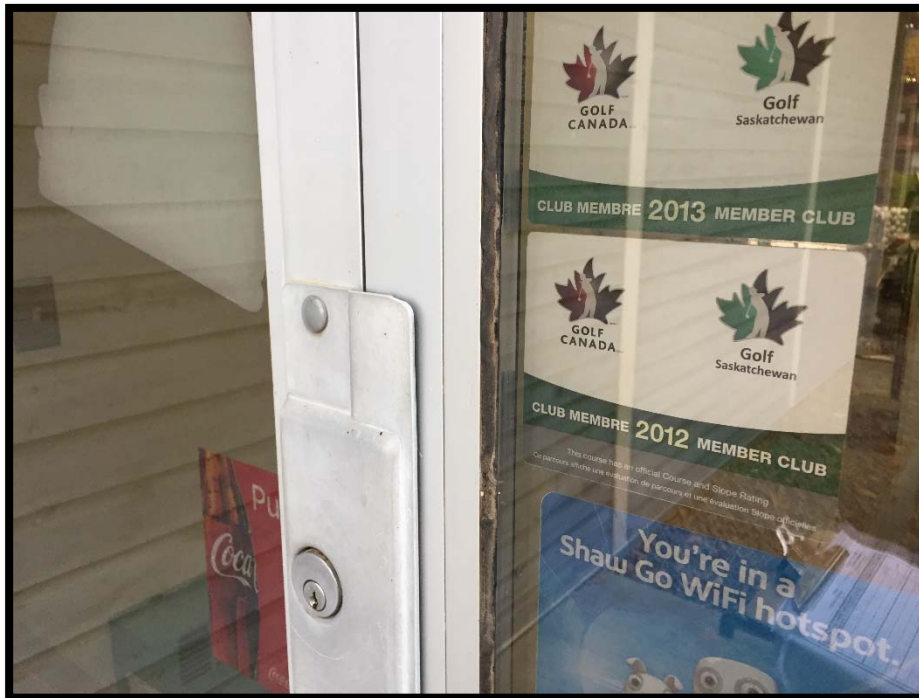
Photograph 4: Asbestos-Containing Black Exterior Window Caulking.
