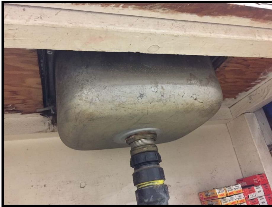
Photograph 1: Asbestos-Containing Gold Sink Undercoat.
