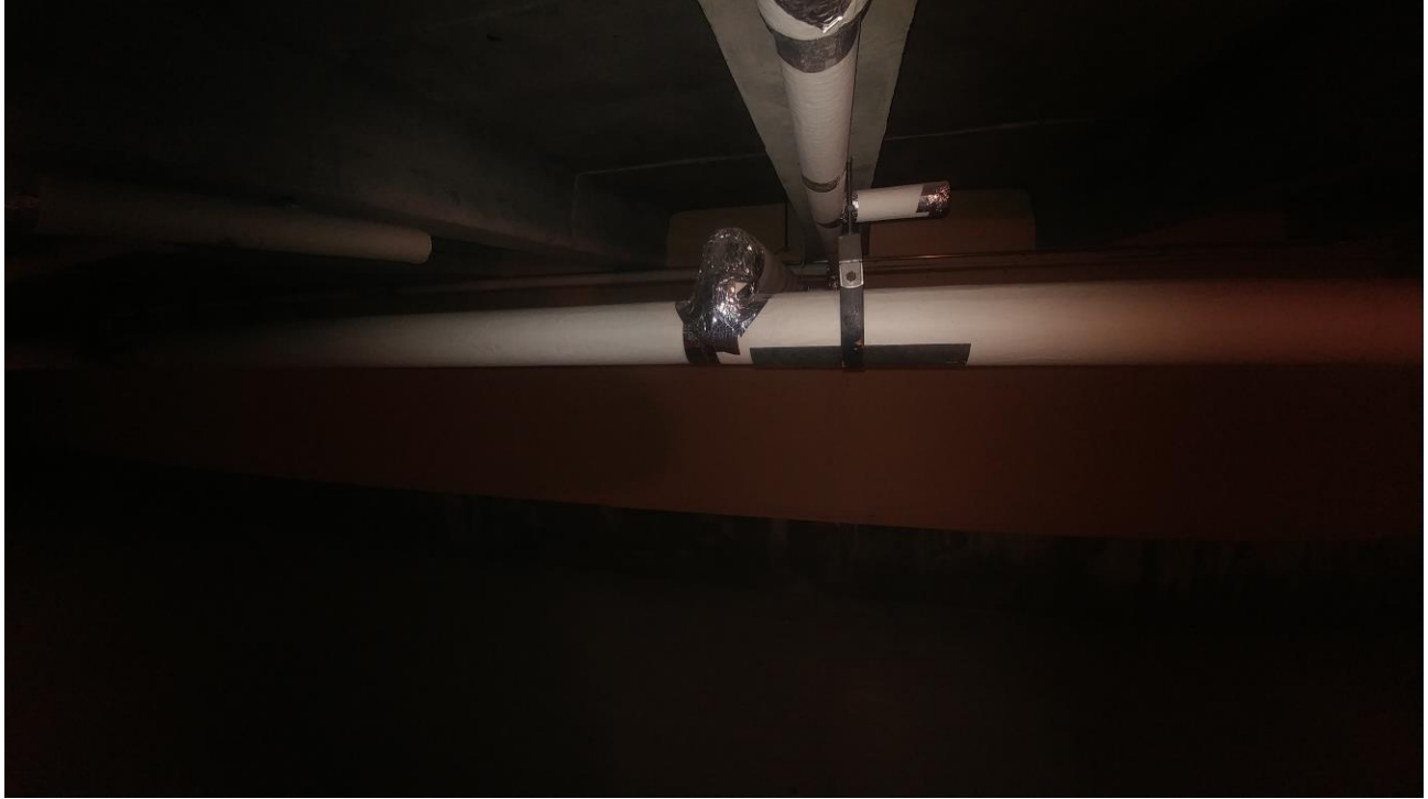
PHOTO 1 – Fiberglass Lineal Pipe Insulation w Fiberglass Elbow in Foil Wrap
