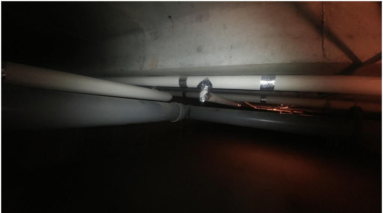
PHOTO 2 – Fiberglass Lineal Pipe Insulation & PVC Drainpipe
