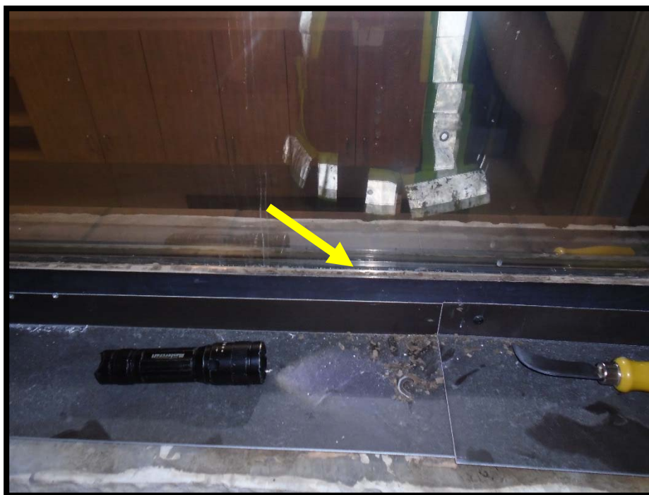
Photograph 1: Asbestos-Containing Grey and Black Window Caulking
