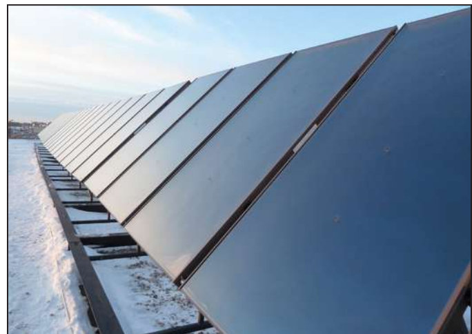
Solar Panels at Lawson Civic Centre
