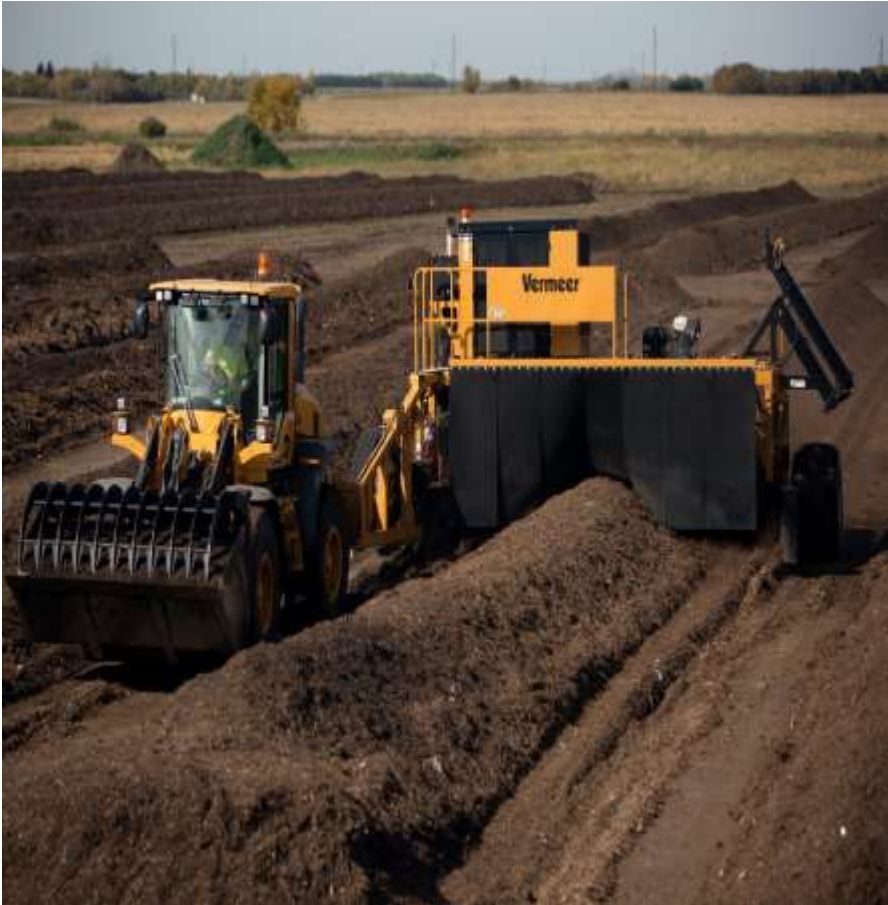
Compost Windrow Turner at West Compost Depot
