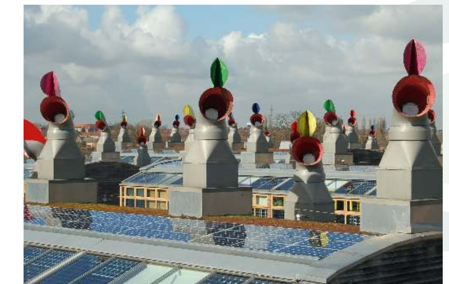
Passive ventilation and solar panels
