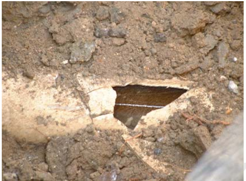
Figure 33 - Hole in Pipe
