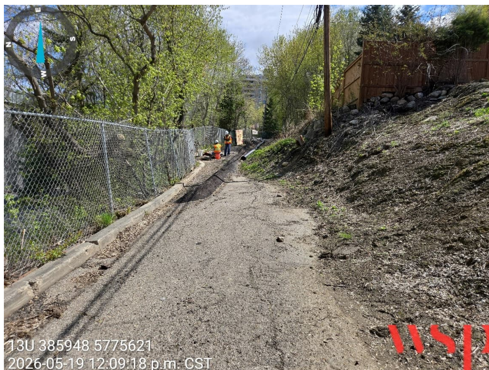
Photograph 2: Looking east down the back alley at the West Failure (May 19, 2026)
