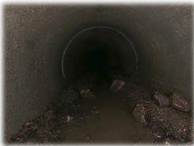
Figure 11: Image of Sediment within Storm Sewer Pipe
