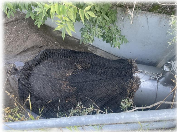
Figure 13: Image of Outfall Net
