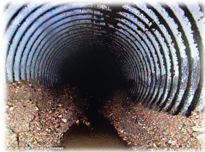
Figure 10: Image of Sediment within Storm Sewer Pipe
