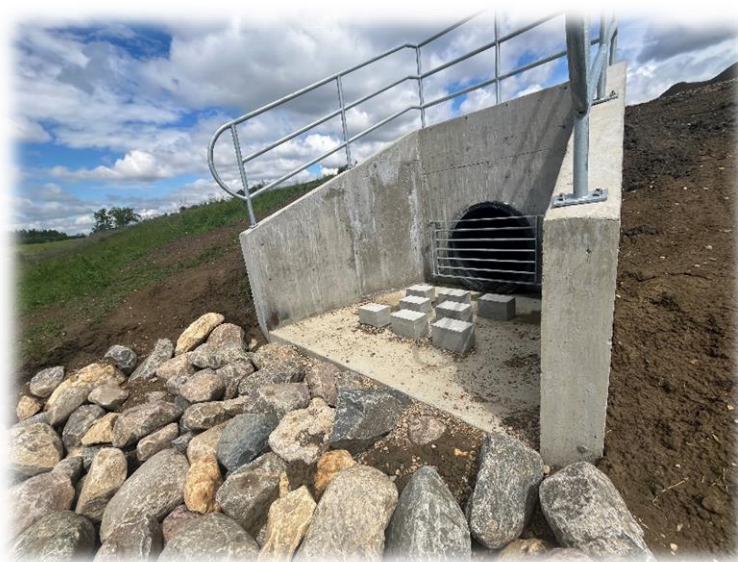
Figure 6: Constructed Storm Water Outfall into Cartwright Pond
